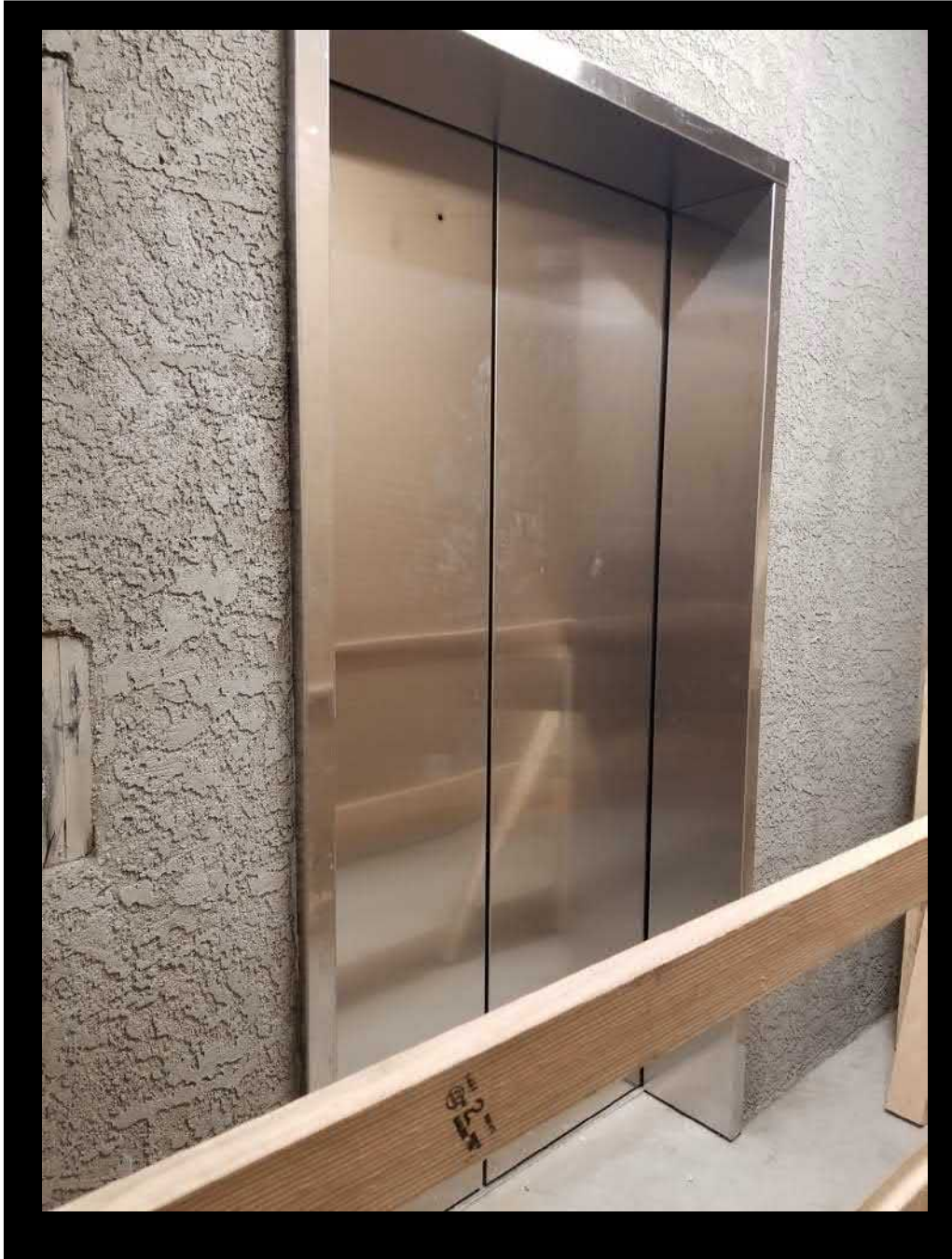
US VETS Elevator (Awaiting State Inspection to Complete)
