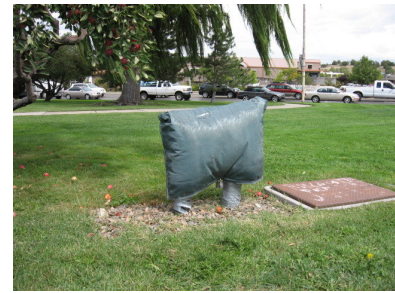
A winterized insulation bag wrapped around a commercial backflow device.
