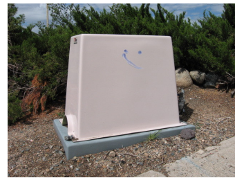
Insulated box installed and locked to protect backflow device from freezing and tampering.
